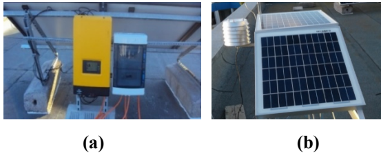
Fig. 2. (a) The DC/AC inverter, and (b) The deployed weather station.
