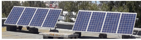
Fig. 1. The 8 pc-Si PV panels.
