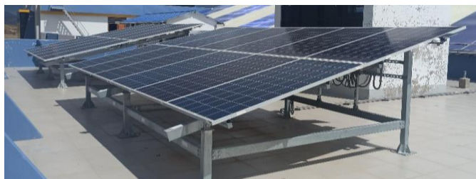
Fig. 2. Photovoltaic solar system installed.
