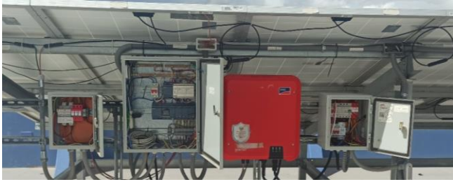
Fig. 6. Data collection instrumentation installed.
