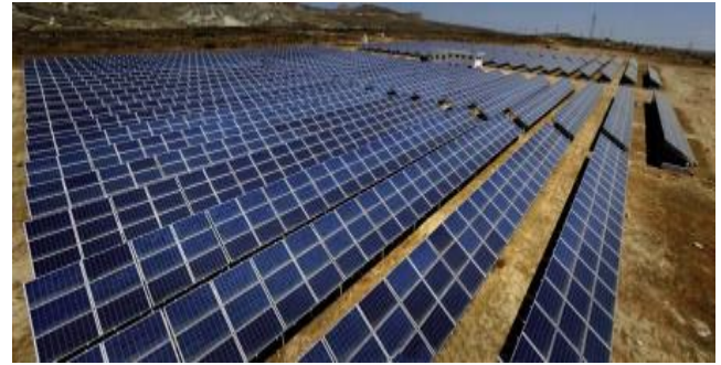
Fig. 5. Serhatkoy PV power plant [19]
