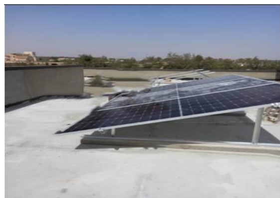
Figure.12. The real hybrid system in the house
