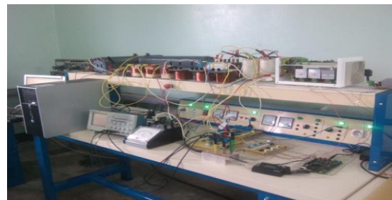
Fig.10. PWM Rectifier With the function of an Active Power Filter experimental test bench
