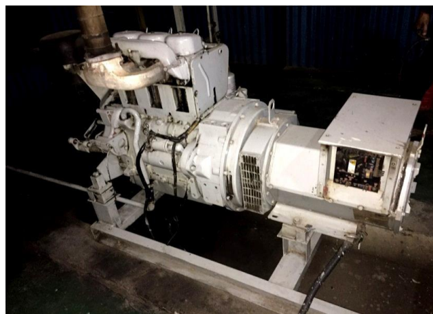
Fig. 4. Existing diesel generator in the Ngadu Ngala grid
