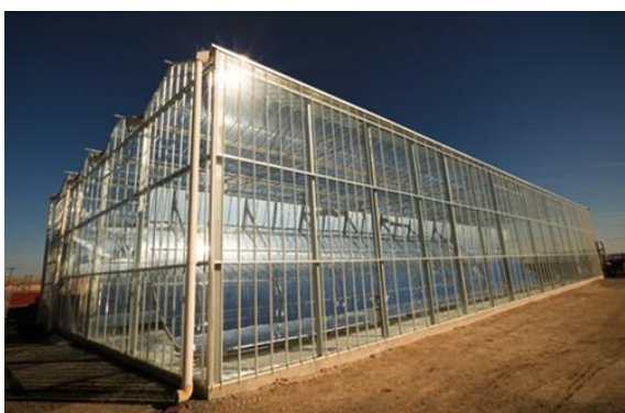
Figure 8. Photo of the solar EOR facility installed in the Amal oil field, Oman (image source: https://en.wikipedia.org/wiki/GlassPoint_Solar ).
