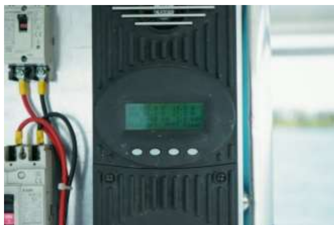
Fig. 7. Charge controller and inverter unit
