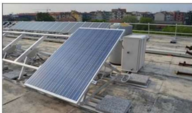
Fig. 6. The PVT system located at Test Facility of the Politecnico di Milano[27]
