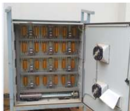
Fig. 3. Box of the resistive loads. This box is installed outside to prevent the overheating of the characterization room as we operate under hot climate.
