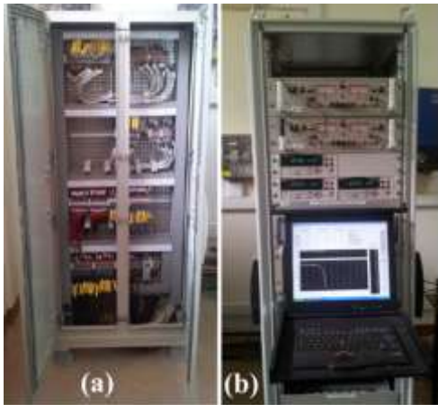
Fig.4. Internal Part of the I-V bench: (a) Patch panel, (b) Electrical bay.
