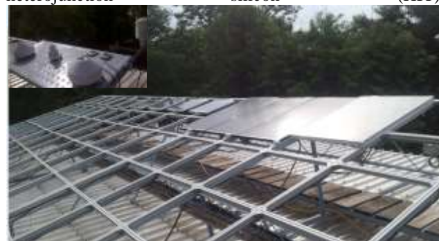
Fig.2. Modules metal structure. The inset picture shows the radiation measurement sensors mounted on a plateau that is tilted at the same angle as the modules.
