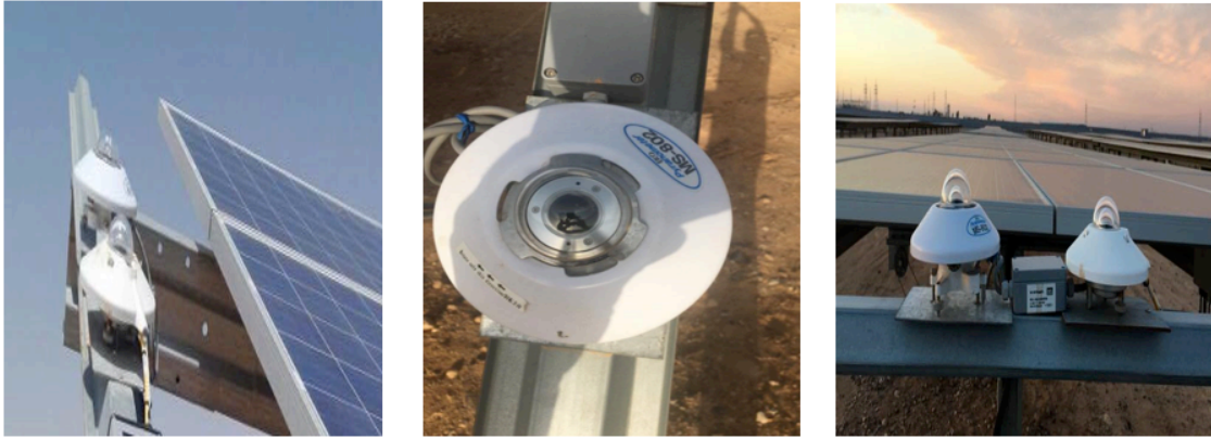
Fig. 2 SMP10 Pyranometer installed on OPVP
