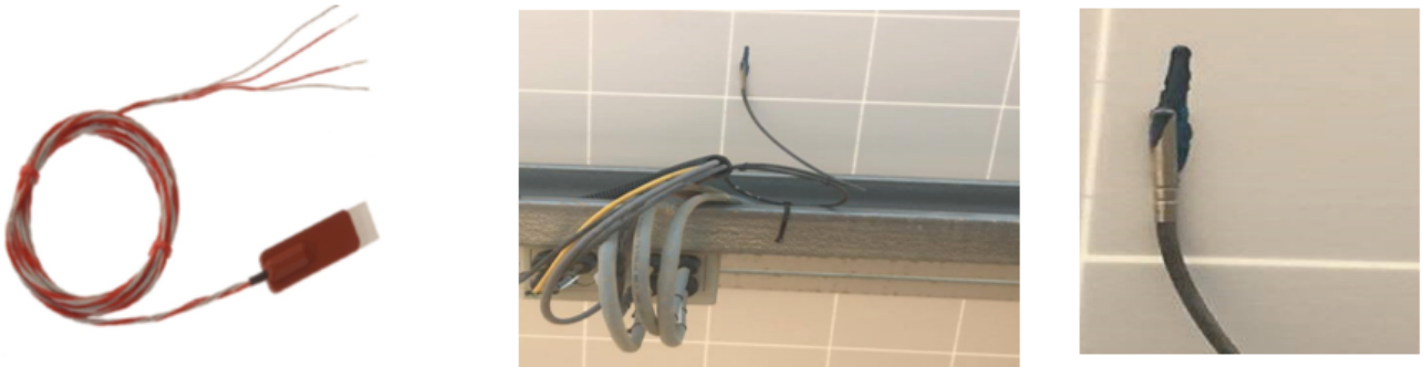
Fig. 4 The module temperature Sensors (PSPS) installed on OPVP
