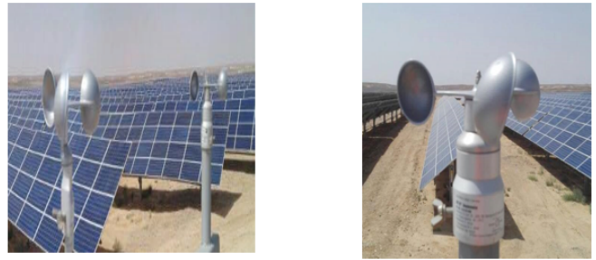
Fig. 1 The Anemometer installed on OPVP
