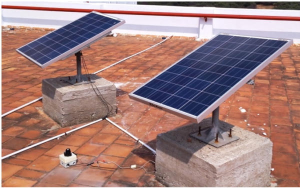
Fig. 9 Solar PV string setup for real time analysis
